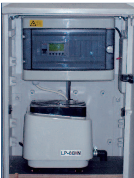
Switch cabinet with control unit and aeration pump
